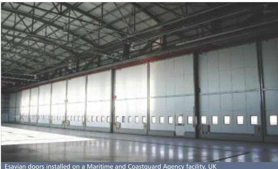
Esavian doors installed on the Future Strategic Tanker Aircraft hangar in the UK
